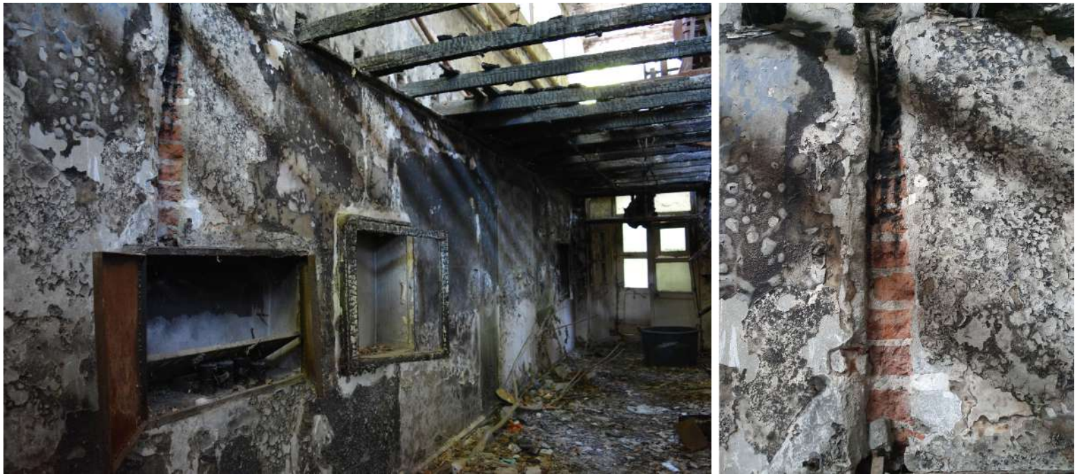
Figure 4.34 Brickwork of the wall is visible from under the plaster.
