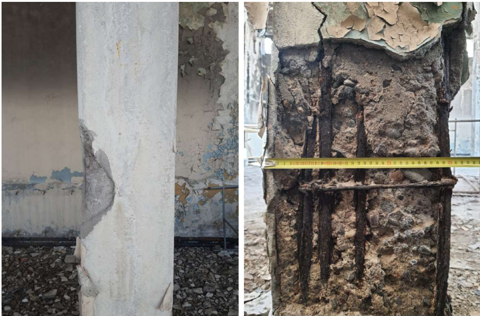
Figure 4.36 Structural decay of the columns in the cinema hall
