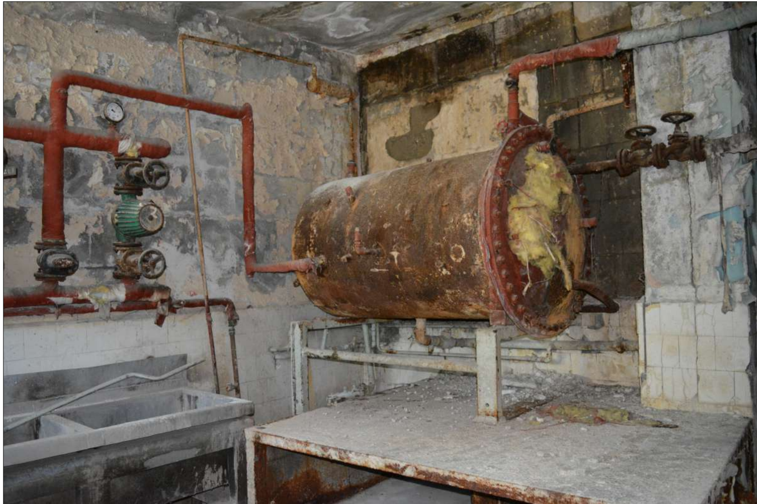
Figure 4.11 Water tank of the kitchen
