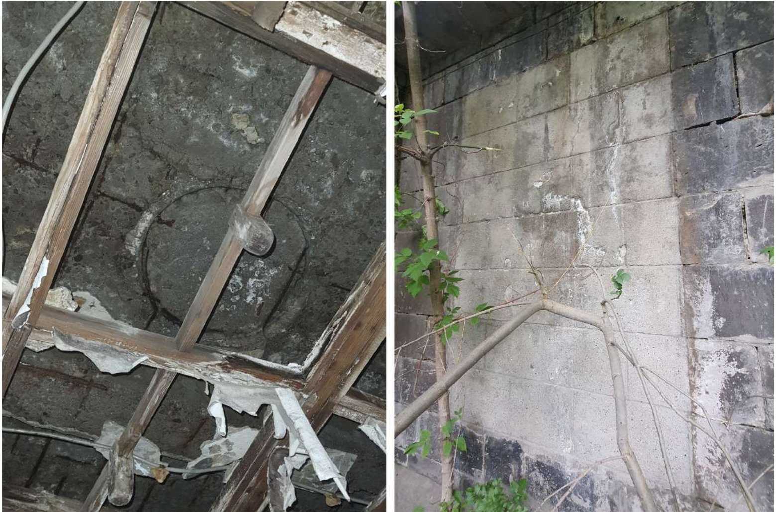
Figure 5.1 Traces of the closed chimney in club section and opening on the northern facade
